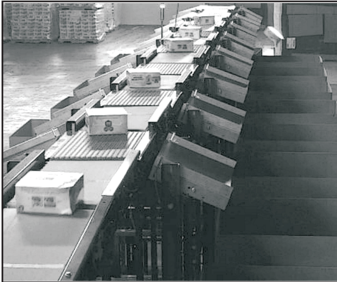
MAI Parcel Handling Sortation Systems
